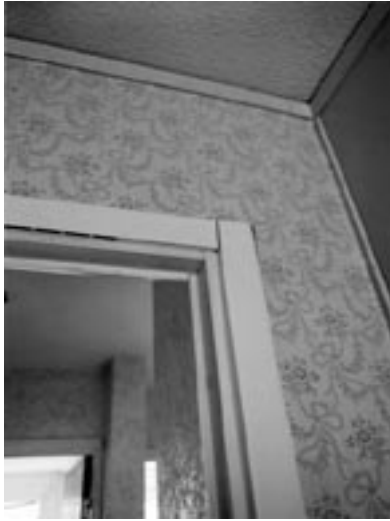
Detailing. Plastic cover strips around doors. Thin strips hide the poor fit of prefab wall units.
