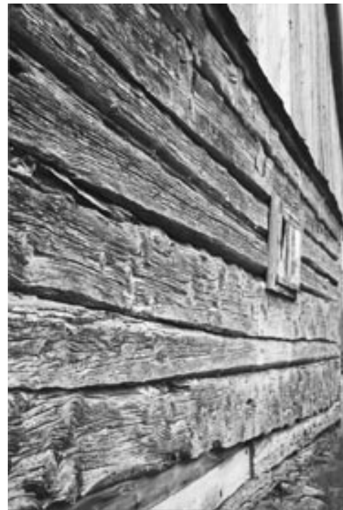
Façade, Åskhults by. Each individual plank seems to speak of its origins.
