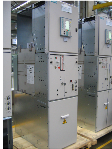
Fig. 1. A typical electric switchboard (Wikimedia, https://commons.wikimedia.org/wiki/File:Medium_voltage_panel.jpg ; Retrieved 05/01/2021)
