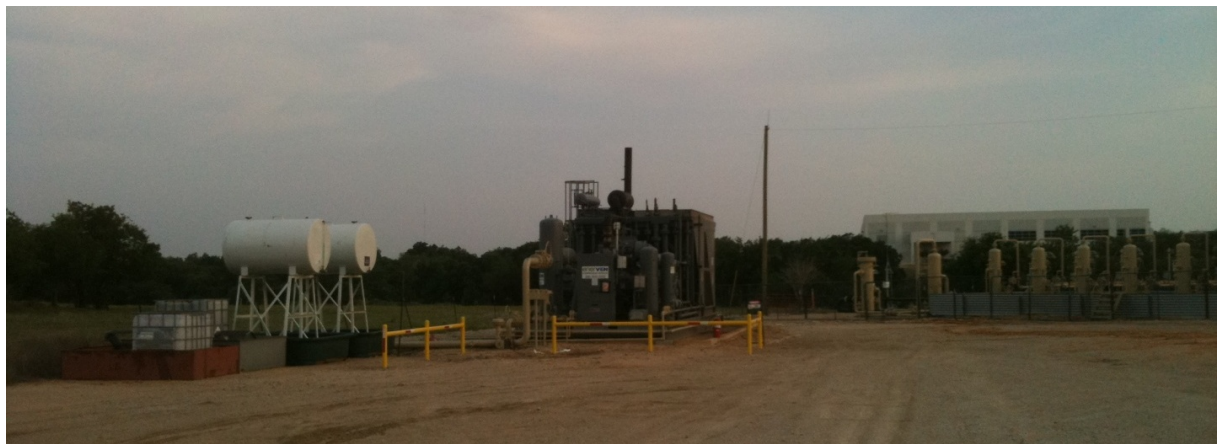
Figure 84 The compressor and separators near Meacham Blvd.
