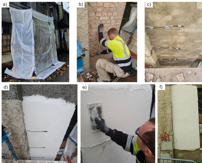
Fig. 3. Application steps for the ACM-system, including a) Weather protection used during the application phase to prevent weather induced stresses. The process involved b) Preparation, removal of the existing coating mortar, and cleaning of the substrate, c) Application of undercoat/base mortar, d) ACM, and e) A first layer of outer mortar with reinforcement mesh, f) Final appearance of the test wall after removal of the weather protection.
