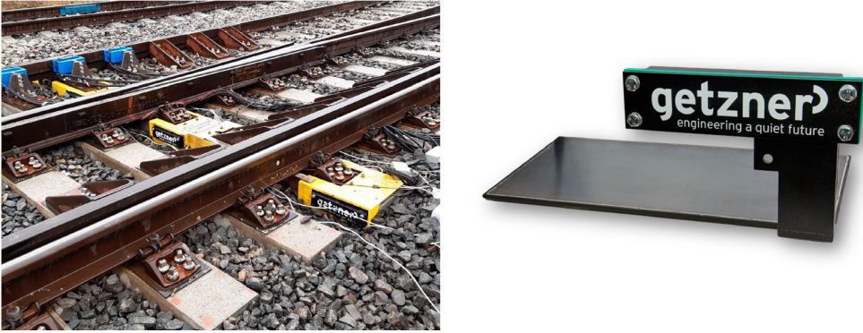
Figure 3. Sensor Sleeper in track (left) and individual sensor (right).
