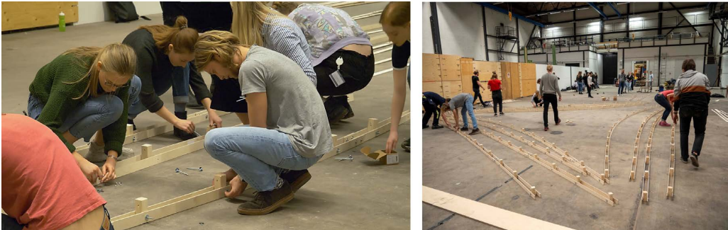
Figure A.22: The laths in the bottom layer are connected to the timber blocks during the 2019 workshop. Left, a closeup of the process and to the right the connected laths are laid out before connecting the top layer.
