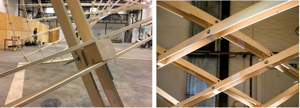
Figure A.1: The nodes of the asymptotic timber grid shell built during the 2019 workshop. The timber blocks connect the laths in two layers, making it possible to lock the mechanism in the erected state. It requires a slot to accommodate the transformation from flat to erected state, as seen in the left picture.
