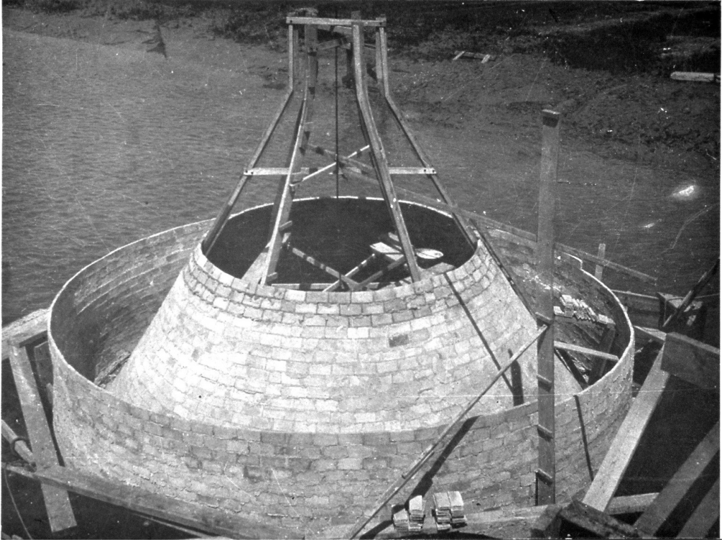
Figure 4.11: Eduardo Torroja using thin brick shells as form-work for the foundations of the Sancti Petri Bridge, 1927.
