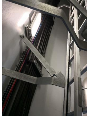
Figure 3.6: Cable bundle inside wind tower.
