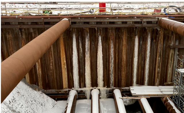
Fig. 18. Leakage from the joints of SPW (Bozkurt, Sinem. West Link project, Gothenburg. 16 Feb. 2021. Author's personal collection).
