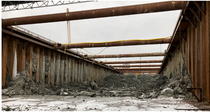
Fig. 11. The final excavation level of West Link excavation at KM:456+850 (Bozkurt, Sinem. West Link Project, Gothenburg. 16 Feb. 2021. Author's personal collection).
