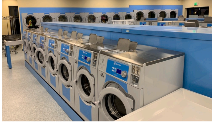
Fig. 1. A snapshot of a public laundry facility [23].
