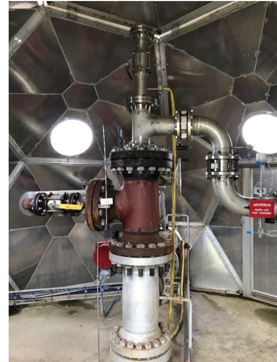
Water, wherein greenhouses gases have been dissolved through the Carbfix method is led back into the ground
