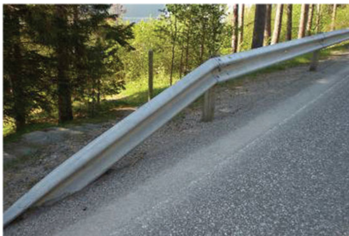
Fig. 4 Turned down guardrail terminal. (Photo: Marianne Gjerde (2008))
