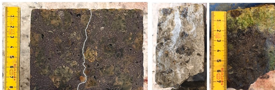
Fig. 10. Carbonation detection on core C1. Left: freshly cut concrete core sprayed with rainbow indicator; Right: crack face sprayed with a rainbow indicator (left side: cut surface; right side: outer cylinder surface). (For interpretation of the references to colour in this figure legend, the reader is referred to the web version of this article.)
