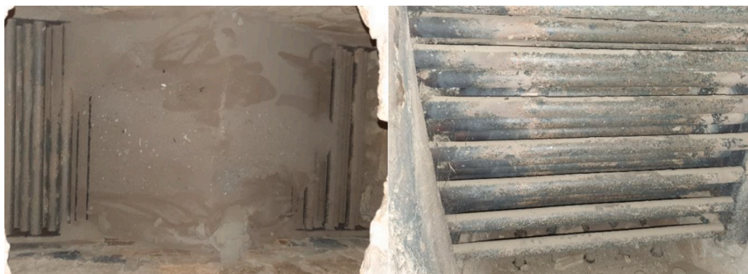
Fig. 6. Two images of a fluidized heat exchanger (from the top to the left and from the side to the right) where a lump had formed at the top of the tube bundle.
