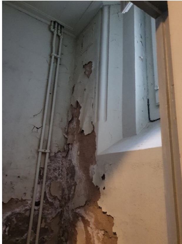
Figure 8. Example of the moisture-related damage at the interior of the Örgryte New Church: weathering of the internal coating mortar (plaster) and paint, and salt efflorescence. Photo: the authors.
