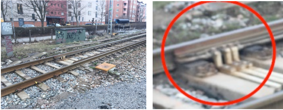
Figure 28 A 1:15 switch with a zoom-in of the connection between the drive and the switch rail. (B Paulsson)
