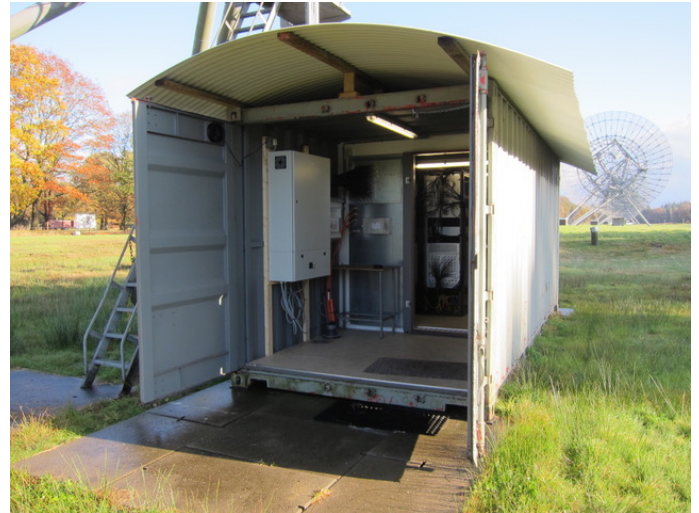
Fig. 14. Telescope cabin, an EMC-shielded Faraday cage in a shipping container.
