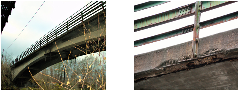
Figure 3.1: Gullspång bridge: view of the bridge before demolition (left) and exposed tensile reinforcement bars and spalling in an edge beam (right). Photos courtesy of Ignasi Fernandez
