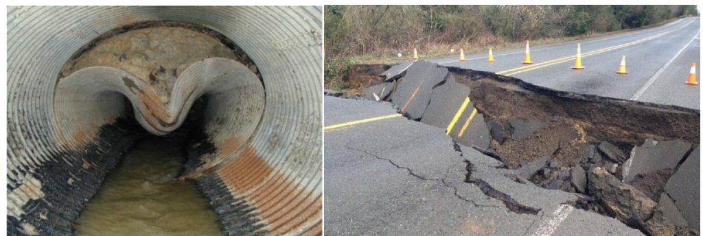
Figure 1. Left: culvert collapse on I-480 in Cleveland (USA) in 2001 [11]. Right: collapse of a culvert in Oregon (USA) in 2016 [12].
