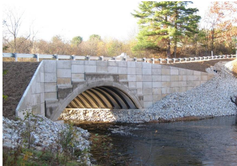
Figure 2. Royal River Bridge in Auburn (USA) with a span of 11.6 m, composed of 13 concrete-filled FRP curved tubes [20].
