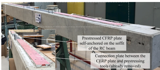
Fig. 2. Self-anchored prestressed CFRP plate on the RC beam (specimen B3) after removing the stepwise prestressing tools [32].
