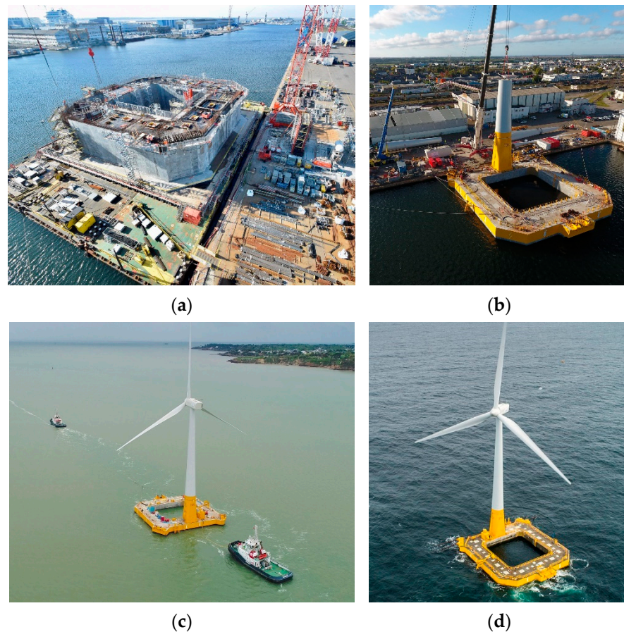
Figure 17. Construction and installation of the Floatgen turbine: (a) construction site for the substructure in Saint-Nazaire harbour, (b) turbine installation, (c) towing of the pre-assemble turbine and substructure, (d) moored and operating floating turbine at the Sem-Rev offshore test site off the French Atlantic coast. (a–c) Credit: IDEOL/ABOVE ALL, reproduced with permission, (d) credit: Valery Joncheray, licensed under CC-BY-SA 4.0.
