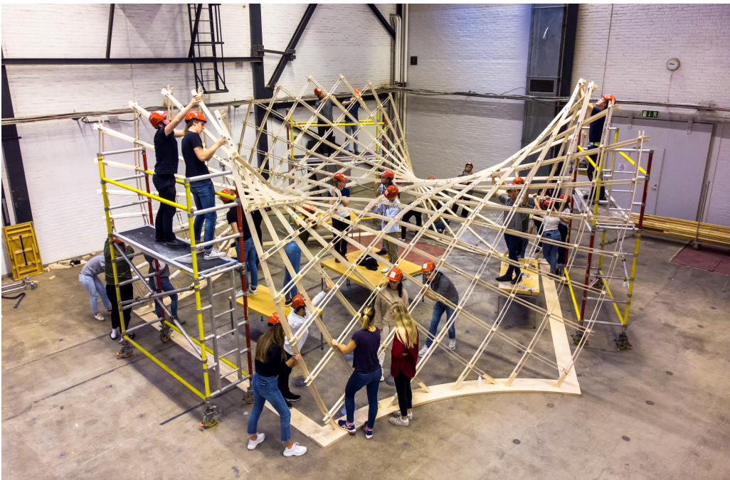
Figure 2.29: Asymptotic grid shell under construction, built with students in the course Parametric Design - Digital Tools with bachelor students at the Architecture and Engineering program in 2019. The author was the part of the design team together with I. Näslund, J. Isaksson, H. Moubarak and C. J. K. Williams
