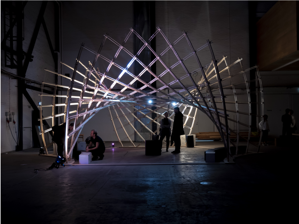
Figure 2.30: Asymptotic grid shell as an exhibition space, built with students in the course Parametric Design - Digital Tools with bachelor students at the Architecture and Engineering program in 2019. The author was the part of the design team together with I. Näslund, J. Isaksson, H. Moubarak and C. J. K. Williams
