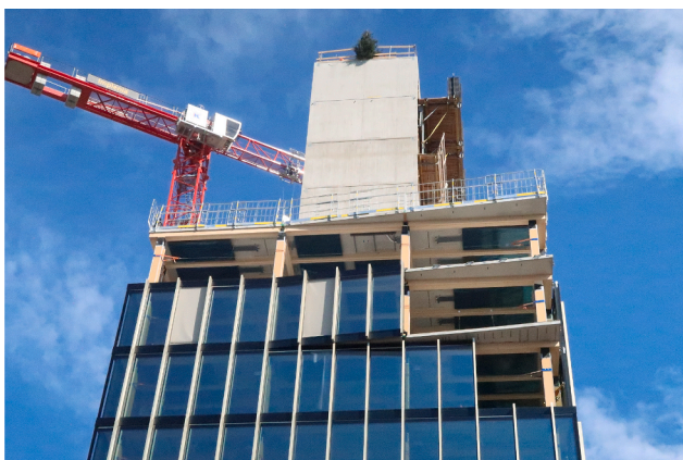
Fig. 2. View of the building Arbo during construction with already completed concrete core and subsequent timber construction.
