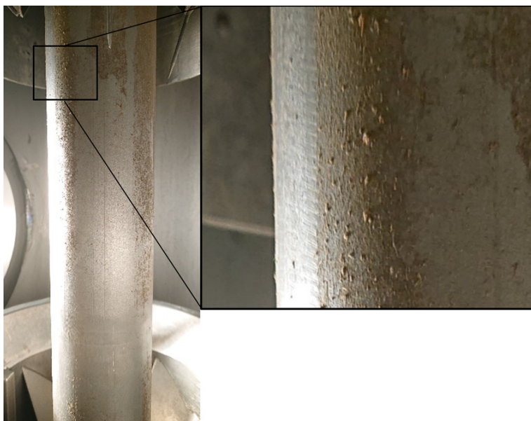
Figure 12: Traces of calcium carbonate scaling found on the evaporator tube after the pre-experiments. The scales were subsequently dissolved and removed using a sulphamic acid solution.
