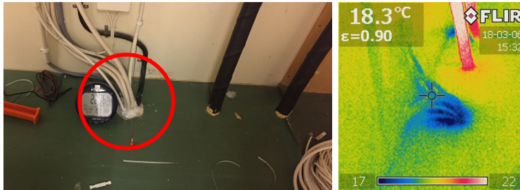
Figure 5.6: To the left is a photograph and to the right is a thermography of air leakage location L1. The air is leaking through a penetration through the floor construction in which electrical wires are installed.
