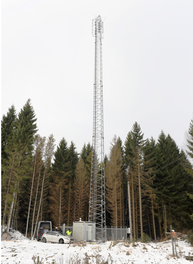
Figure 5.2. Photo of the radar tower soon after construction. The equipment hut can be seen at the base of the tower. Only the P/L-band system was installed at the time.
