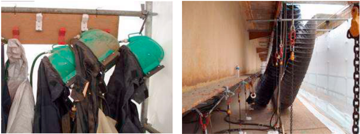
Figure 18: Dressing room and masks for hygiene and safety Containment of the working site to protect the environment, and strong vacuum cleaners.
