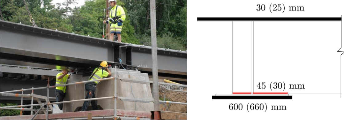
Figure 14. The railway bridge (during construction). Original flange dimensions and the dimensions after HFMI treatment in parenthesis. Red lines indicate HFMI-treated areas.
