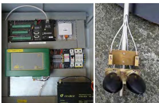
Fig. 3: The pneumatic sensors, Ott CS471 of USGS type, have a compressor (green unit, left) located in the measurement hut. Each compressor is connected to a nozzle (right) via a plastic pipe. Two nozzles are used at the bottom of the well, and one nozzle is located close to the bottom outside of the well. The original black nozzles corroded rapidly in the salty water and were replaced by the ones located just above (manufactured in copper) in October 2016 (see also Fig. 5).
