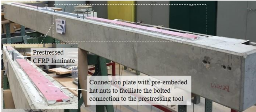
Figure 6. Self-anchored prestressed CFRP laminate on the RC beam after removing the prestressing tool and temporary anchors
