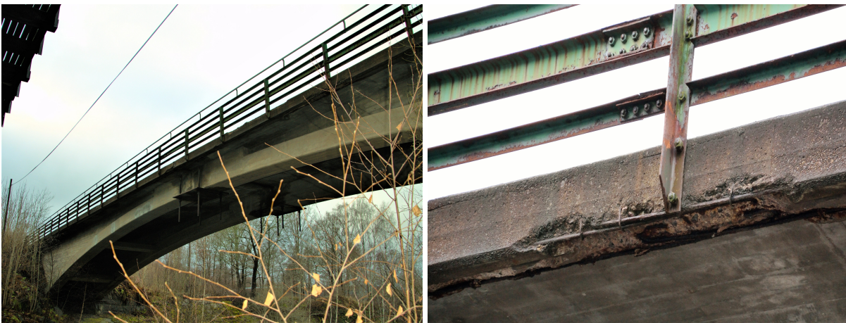
Figure 3.2: Gullspång bridge: view of the bridge before demolition (left) and exposed tensile reinforcement bars and spalling in an edge beam (right).
