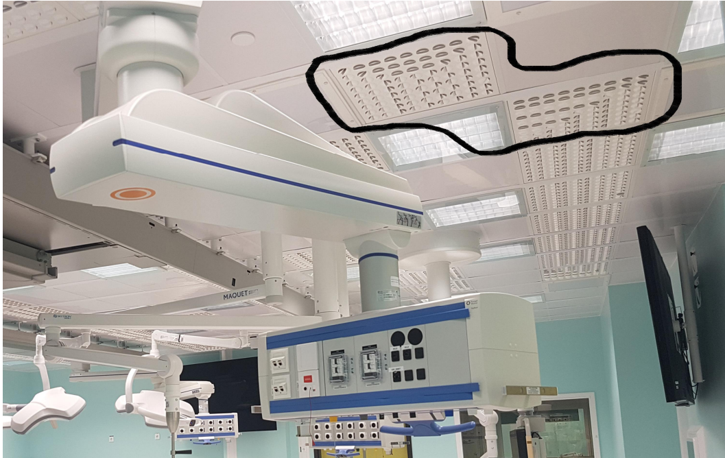
Figure 2.3 A mixing air system at the NKS-hospital. Note that the direction of the supply air nozzles can be readjusted (Photo: J. Nordenadler).
