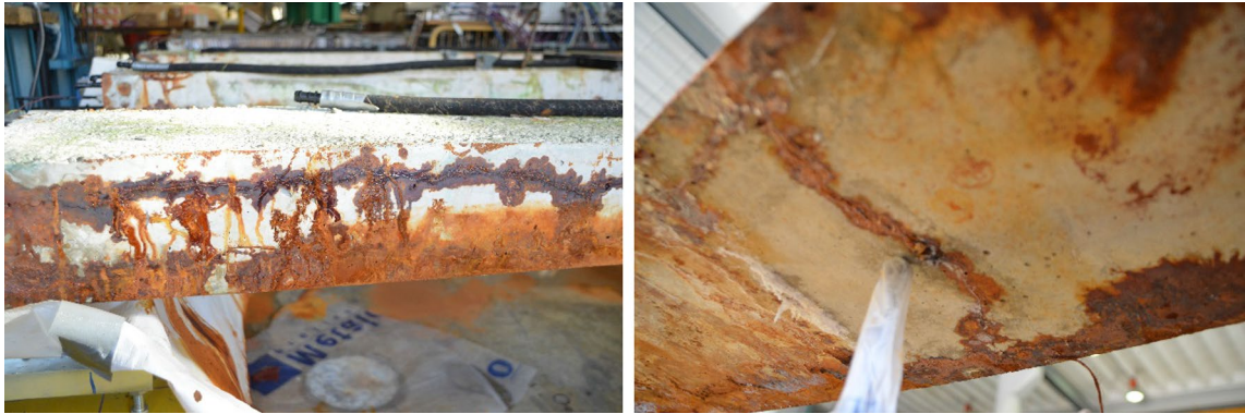
Fig. 7 Deterioration at the end of the accelerated corrosion process: (left) longitudinal and (right) transverse cracks.
