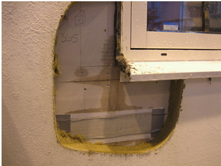
FIG 4. Indicators were placed just below all details behind the façade or exposed surface. The photo was taken after the rain test.
