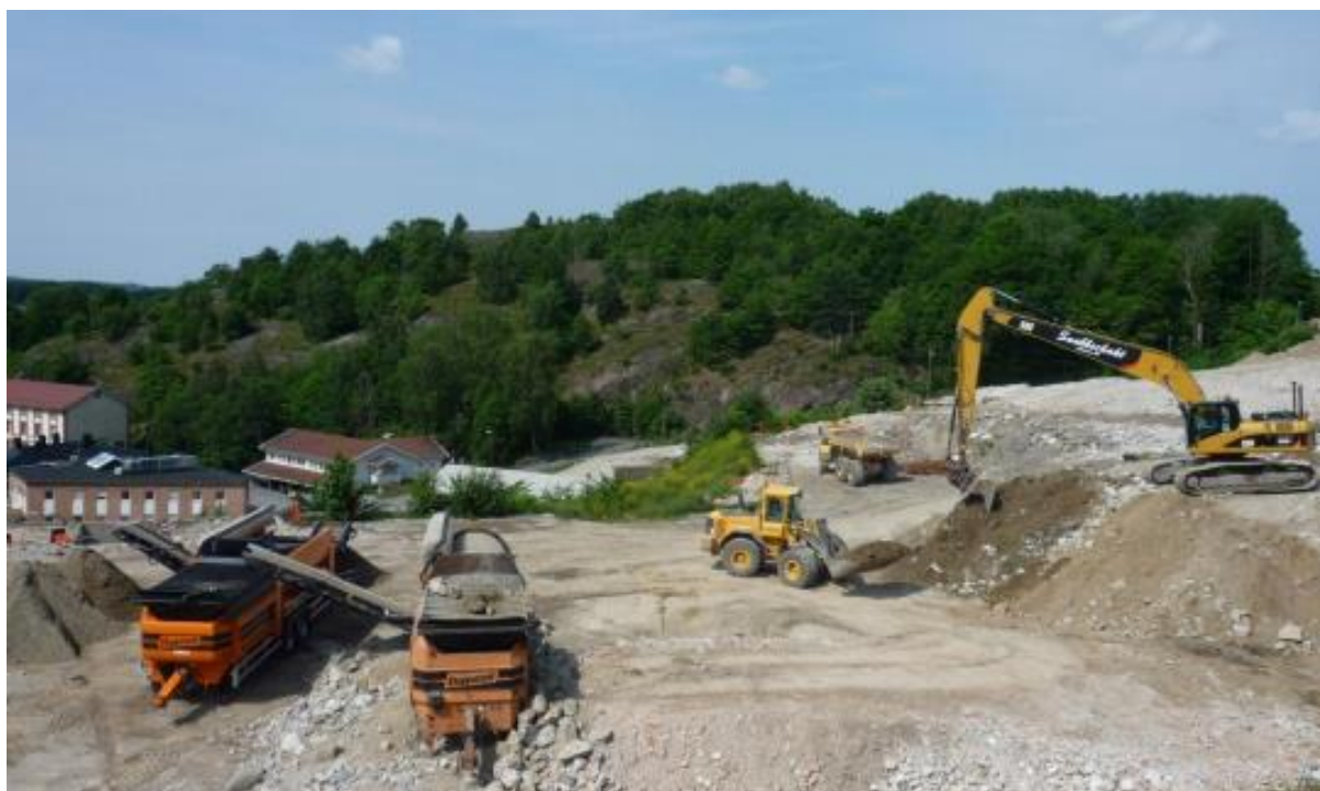
Figure 2-4. Excavation and soil sieving at Hexion site in Mölndal, Sweden. Photo: Åsa Landström (Landström & Östlund, 2011)
