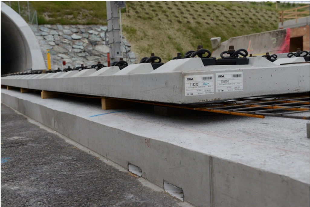
Figure 2.3: The STA system during construction. Note that the asphalt used as a base layer for the track in the photo is normally not used by STA. From STA [5].
