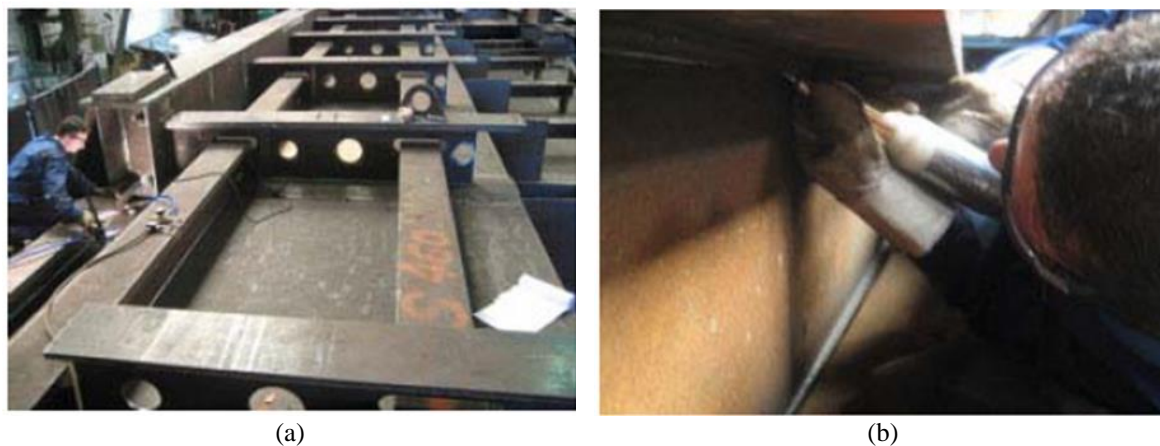
Fig. 3: Schenkendorfstrasse Bridge during manufacturing [10]: (a) fabrication at workshop; (b) Treatment of flange–web welds at workshop
